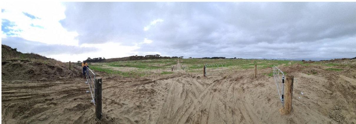
New stock route, paddock gates, and fencelines ready for irrigation to be installed
