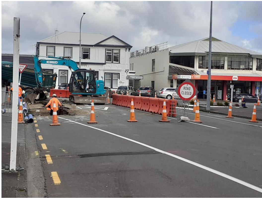
Water supply upgrade work underway on the Queen Street project outside The Warehouse.
