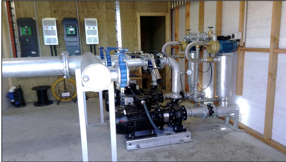
Interior of pump shed showing pumps, pipes, valves and controls.
