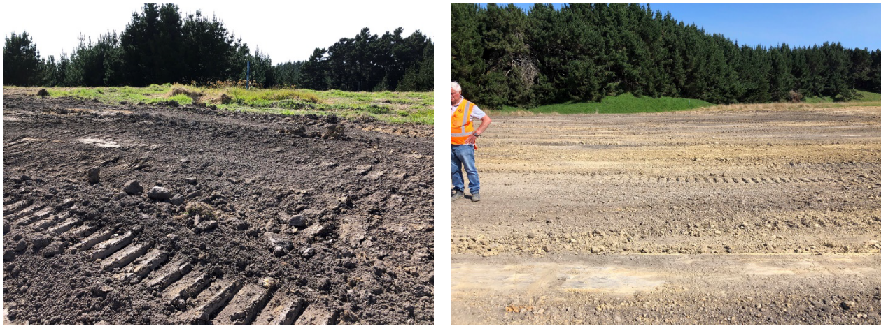
Figure 11-1 Photographs taken on 08 March 2022 showing repairs made to the old landfill surface.
