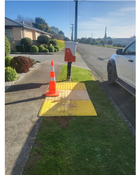
Incident site made safe.
