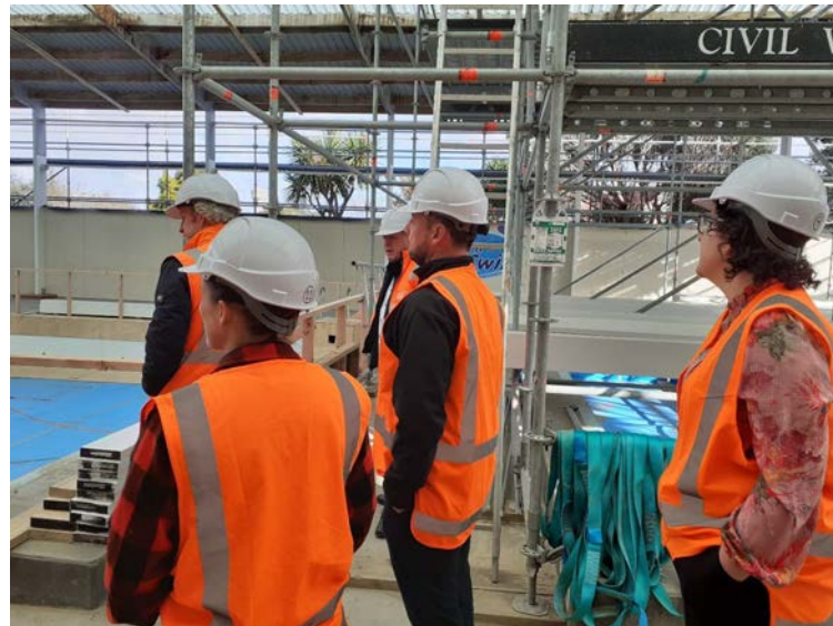
Leadership Walk – Foxton Pool Upgrade June 2023. ELT, RAC and Te Awahou Foxton Community Board attended a leadership walk through the worksite. The attendees had the opportunity to apply a health and safety lens to the worksite and get a greater understanding of contractor management.
