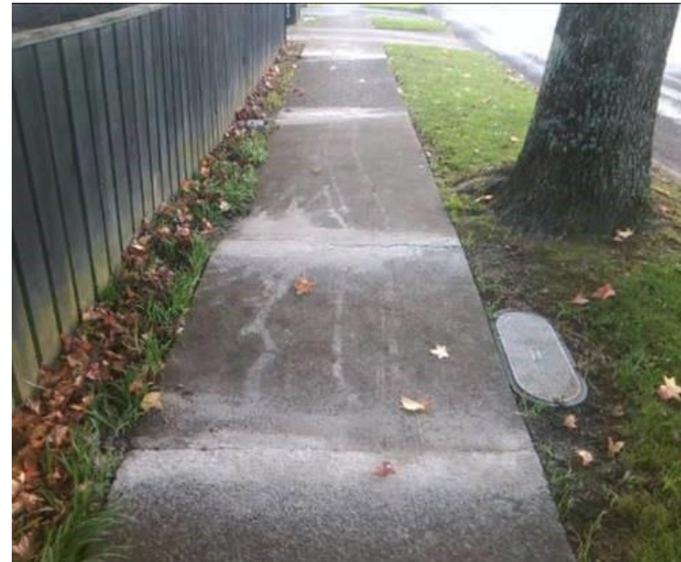
Evidence of grinding repair on footpath.
