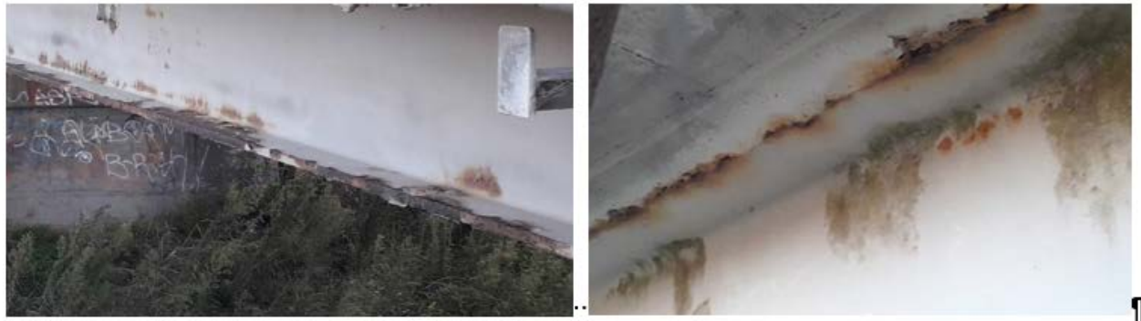
Photos of corrosion on the Manawatu River Bridge.
