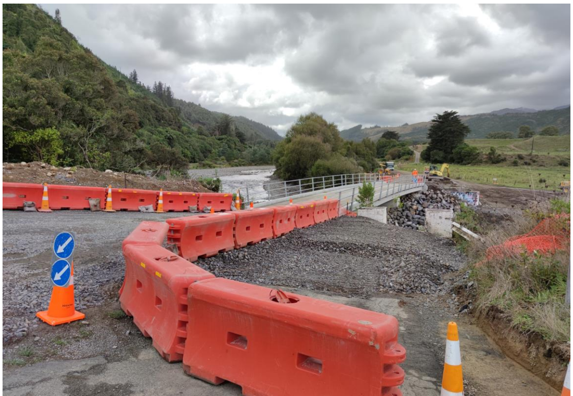
The new bridge open for traffic – The old bridge's abutments are visible next to the new bridge
