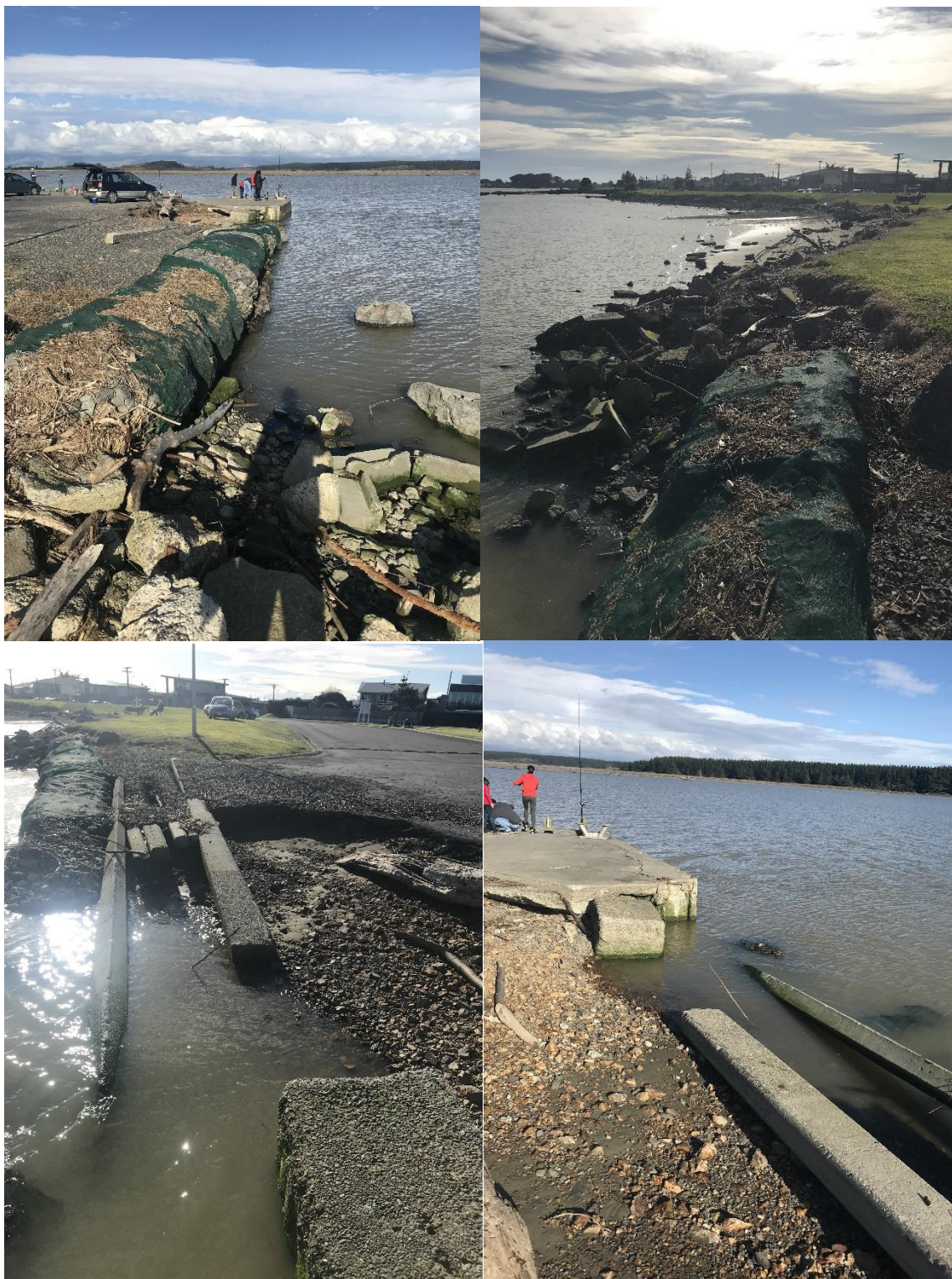
Figure 2.2: Site photographs taken on 19 July 2018 showing the degraded gabion basket wall (upper photographs) and the eroded wharf area (lower photographs)
