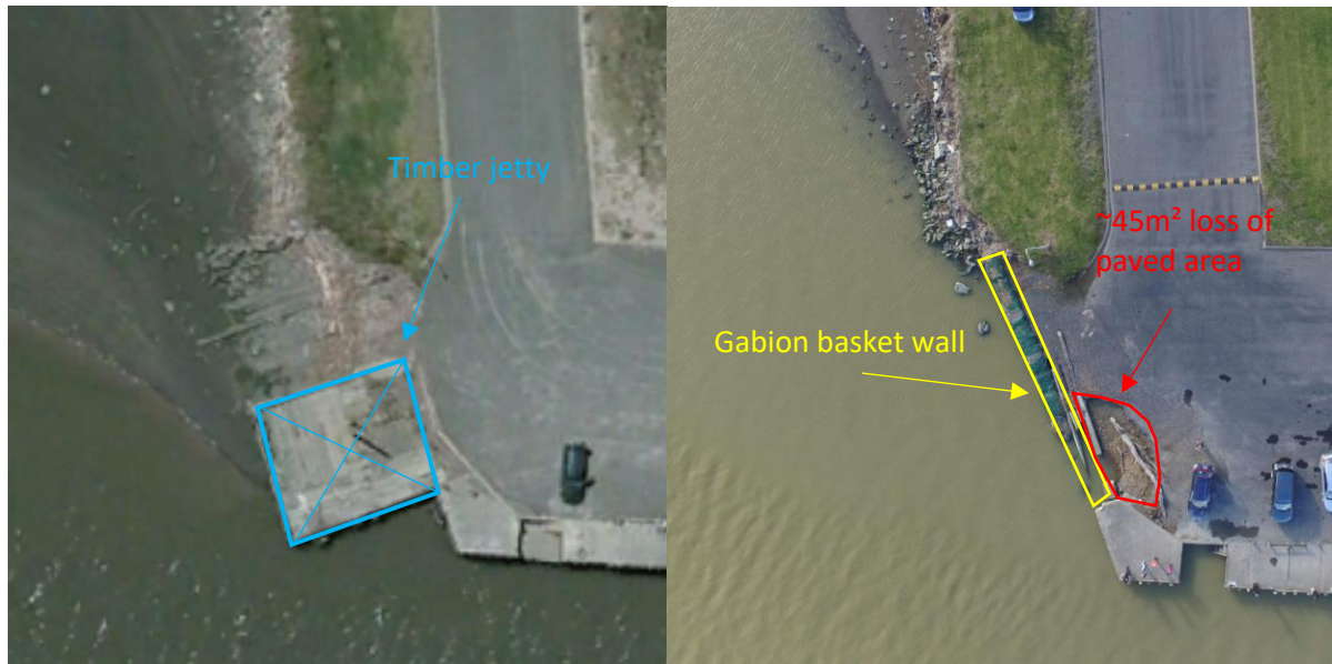
Figure 2.1: Aerial showing historic timber jetty prior to removal (left; January 2010, Google Earth) and erosion at the western corner of Foxton Wharf (right; July 2018, T+T)
