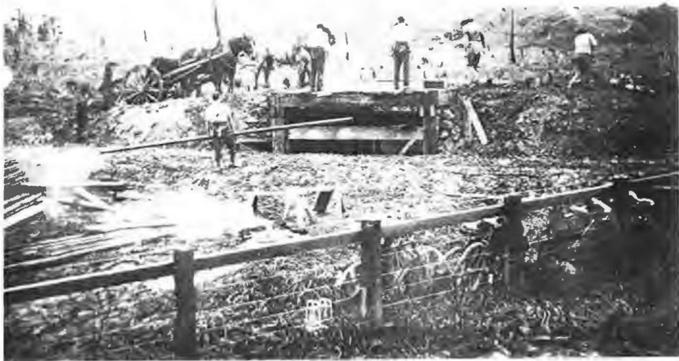
(3) Below: Construction in progress on an unidentified section of the mill. Horsepower was a valuable asset to the builder. Photo: J. McNeile.
