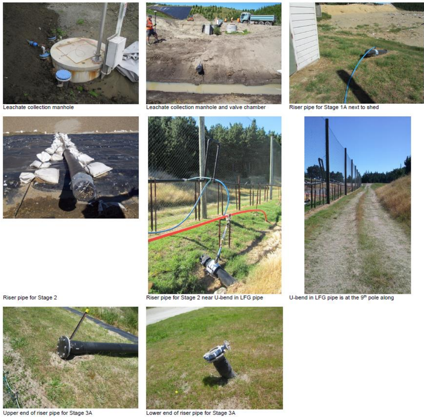
Figure A- 7: Photographs of the leachate collection infrastructure.
