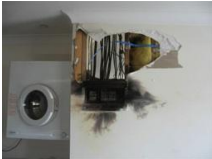
Photo 10: Damage following line drop
