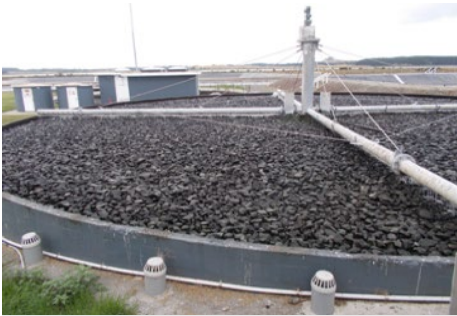
Levin Wastewater Treatment Plant clarifier
