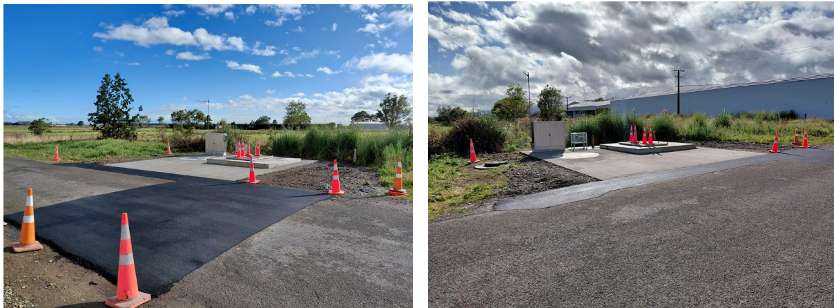
New Bryce Street pump station
