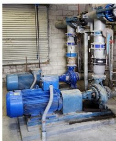
The old 90KW motors and pumps at the POT pumping infrastructure
