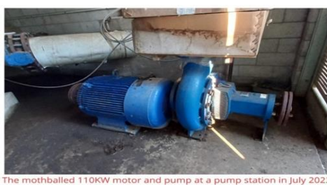
The mothballed 110KW motor and pump at a pump station in July 2023
