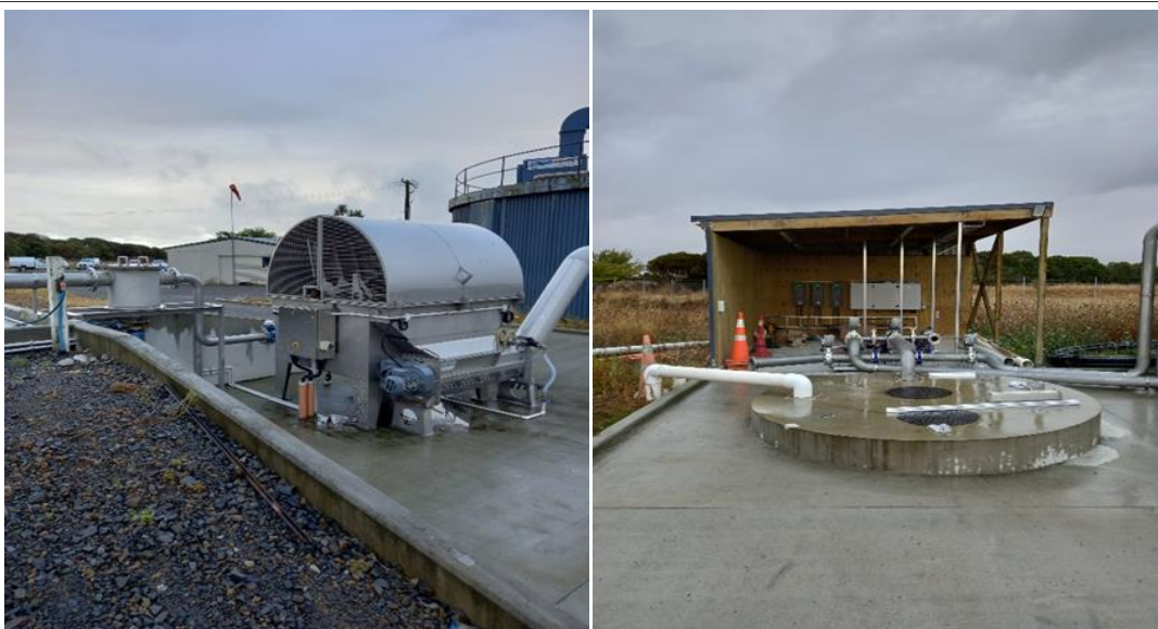
New septage receiving station
