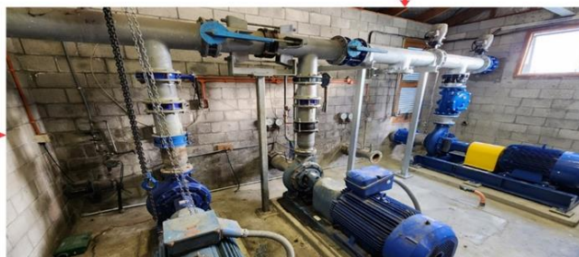
The modified pumping infrastructure at the POT
