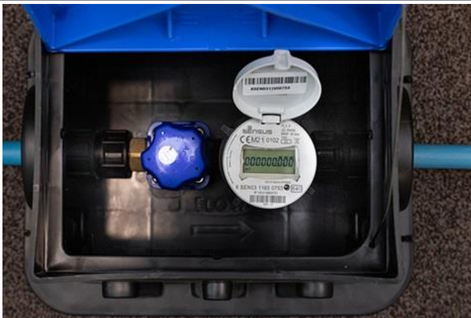
A new water meter being used in water meter programme
