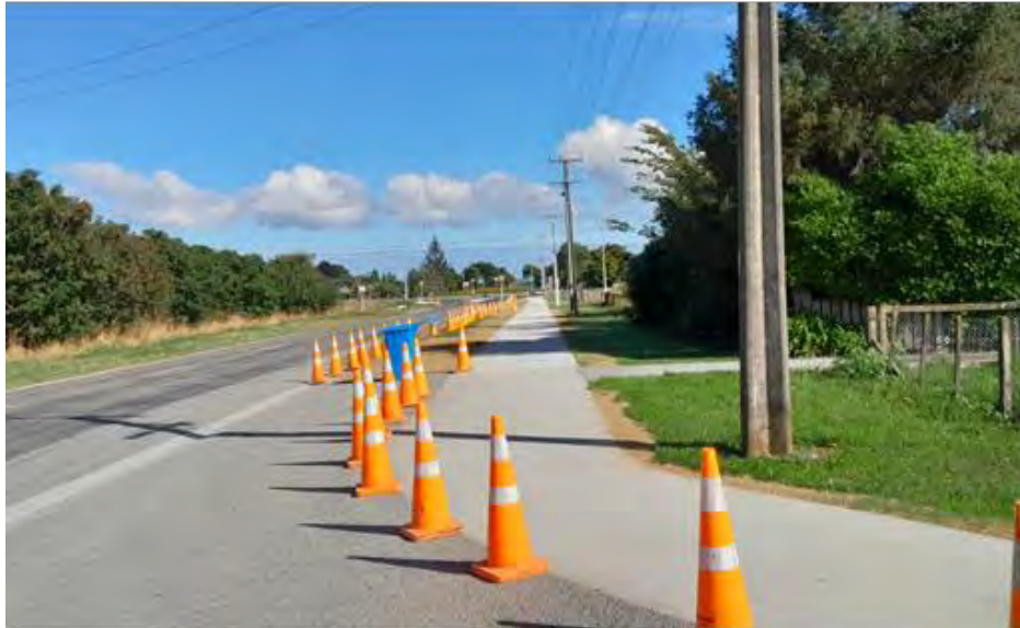
Queen Street East shared pathway is now open for public. Car park chip sealing is complete.
