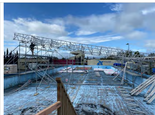
Construction of the temporary painting tent that will be used to paint materials before they are installed.
