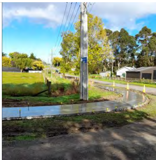
New footpath on Graham Street, Shannon. The new pathway will link Vogel Street to Graham Street. Footpath renewals have started in Julyan Street, connecting to the new footpath in Graham Street.
