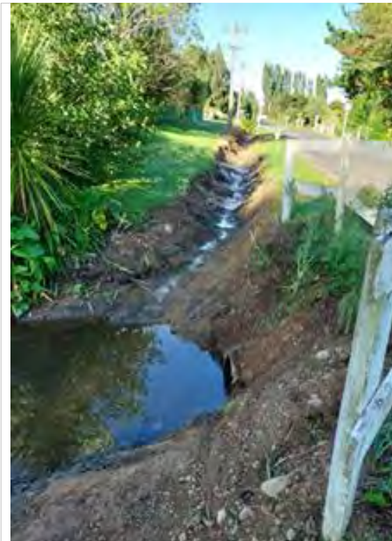
Paranui Road Open drain work has concluded. Open Drain Cleaning is proceeding in Ada Street Shannon. Drain clearing in Te Whanga Road has occurred (pictured below). Residents are delighted with the outcome!
