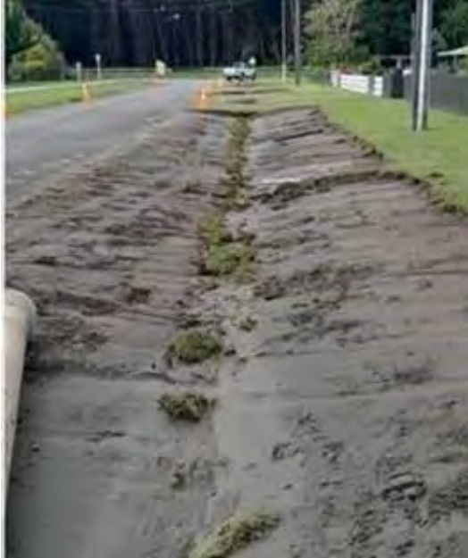
Higgins started the construction and finished the full dig out and prepped at both ends of Kawi Road
