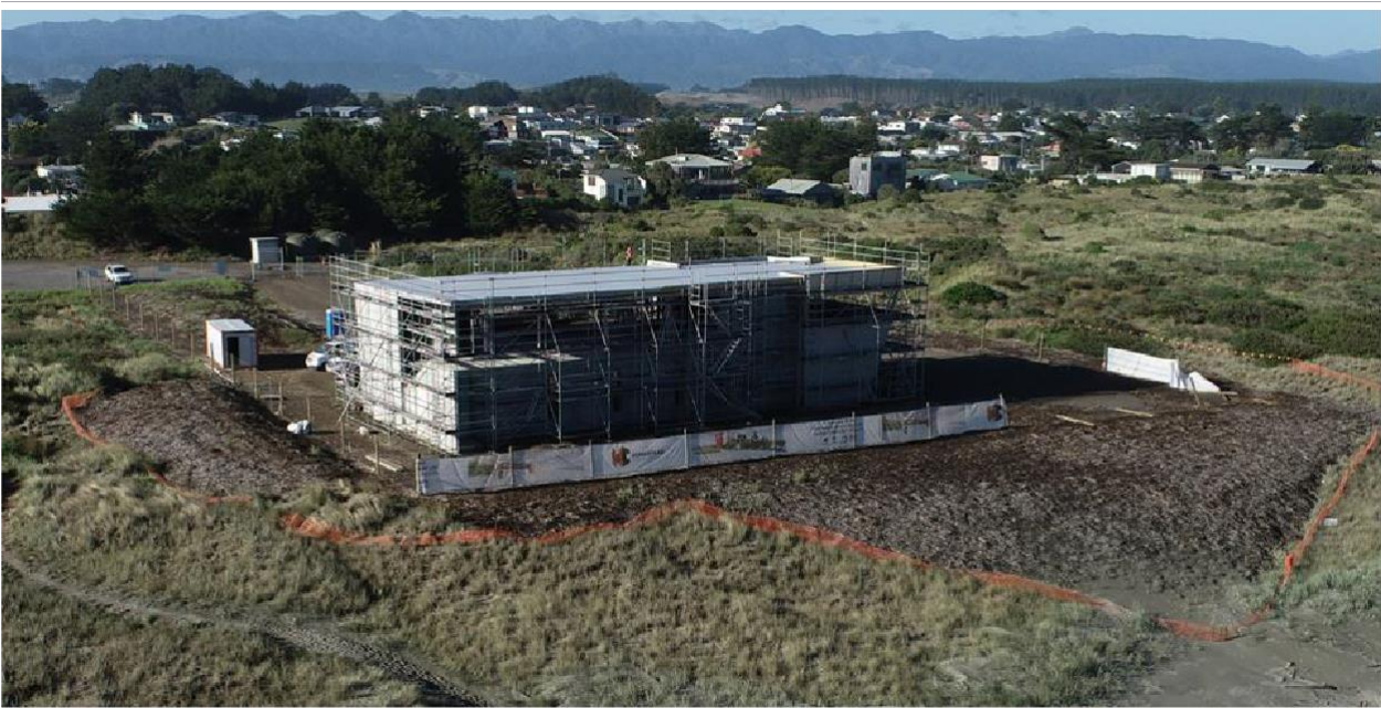
Long Term Plan major capital expenditure projects, Waitāreere Beach Surf Life Club design and build
