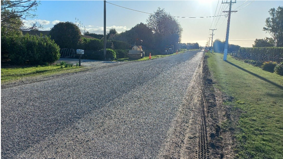
Installed wastewater pipe
