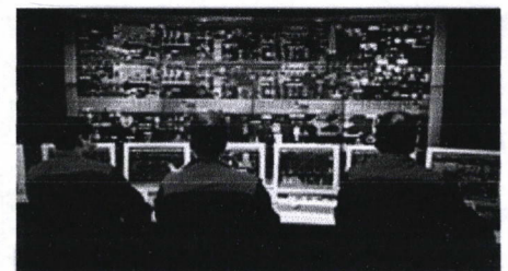
Control room of a typical moving grate incinerator overseeing two boiler lines
