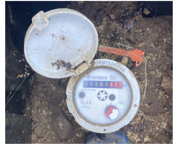
A water meter.
